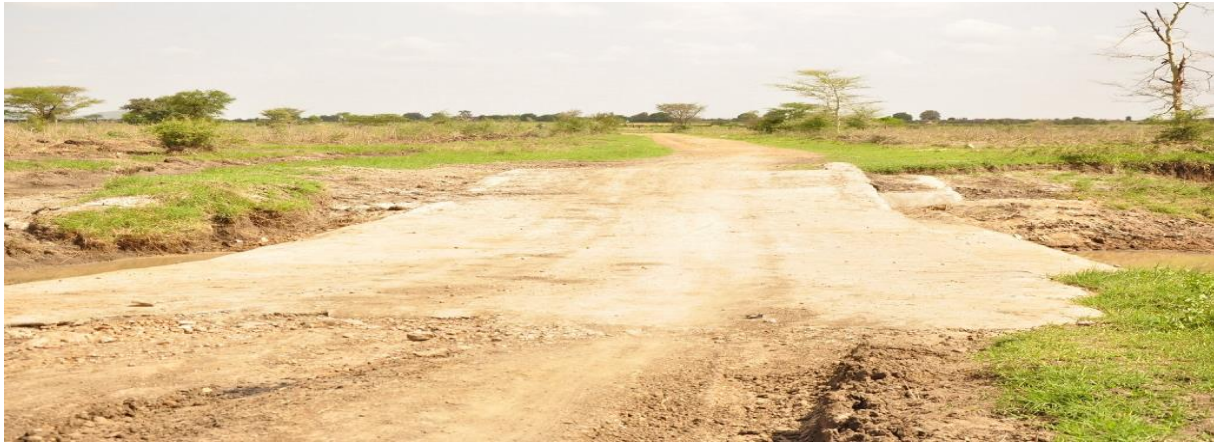
A temporally bridge connecting Nampumpum Sub-county constructed with the NAs intervention after heavy rains washed away the old one
